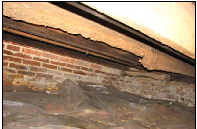
Condition of Joists Under the Church Floor
